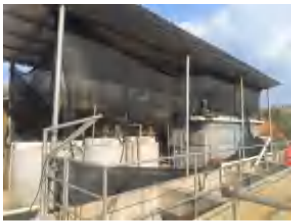
污水处理站-加药区
